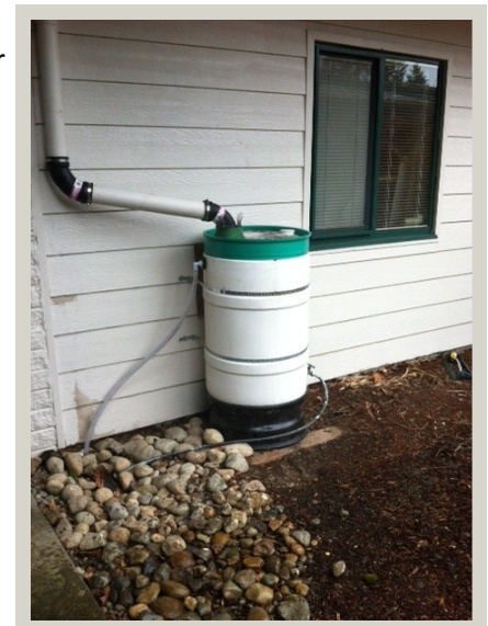
Rain Barrel at CRMS
